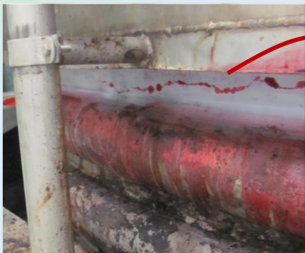
Crack in vessel wall (visible with red die)
